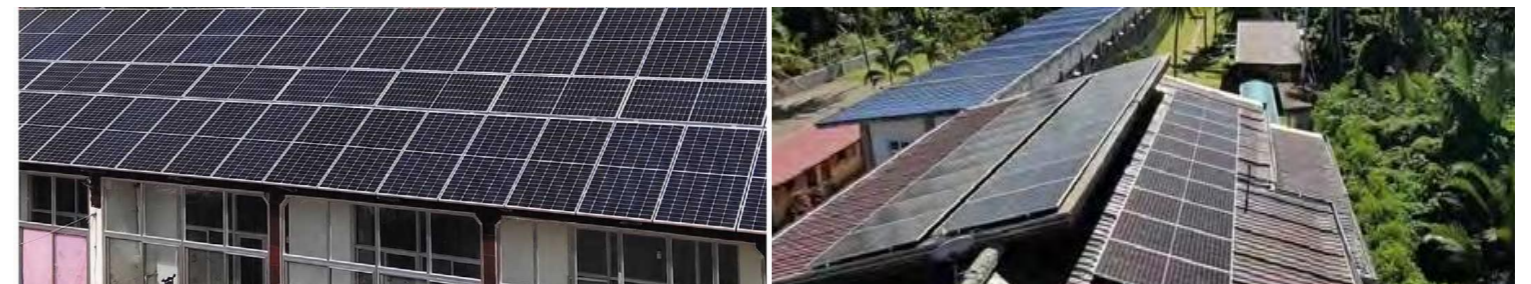
20KW On-Grid Solar System In Indonesia
