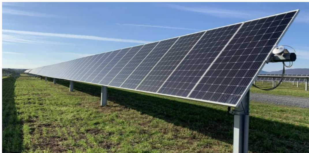
14MW Hy-Grid Solar System
